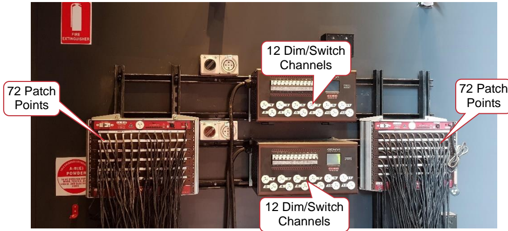
Typical Installation. 144 Patch Points and 24 Dim/Switch channels
